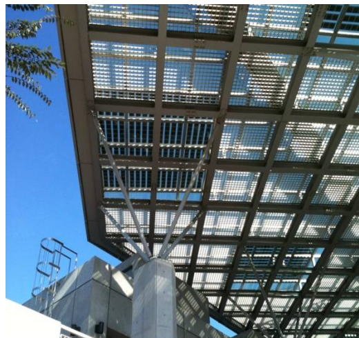
Puduvai Trans solar panel roof top interior
