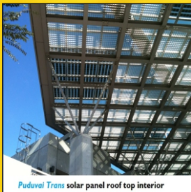
Puduvai Trans solar panel roof top interior
